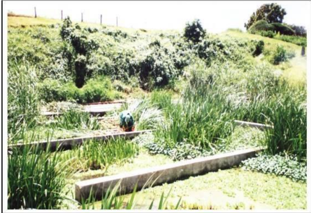
Plate 1. Gravel Bed Hydroponics at Chemomi Factory Constructed Wetland, Nandi Hills
